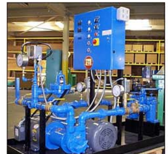
Fuel Oil Handling Systems
